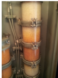
Not maintained dehumidifiers
